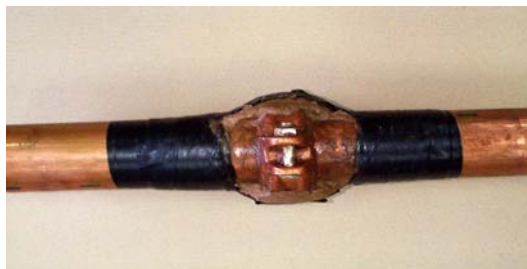
Figure 2: A section of a protected joint showing contoured mastic and overlapped tapes.
